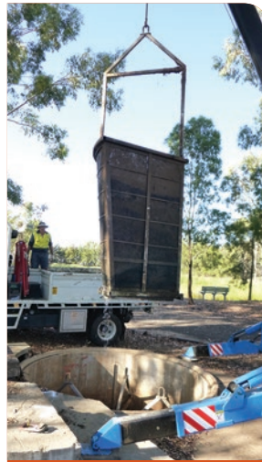
The GPT is emptied on a regular basis to ensure that it is always operating at optimal efficiency.
